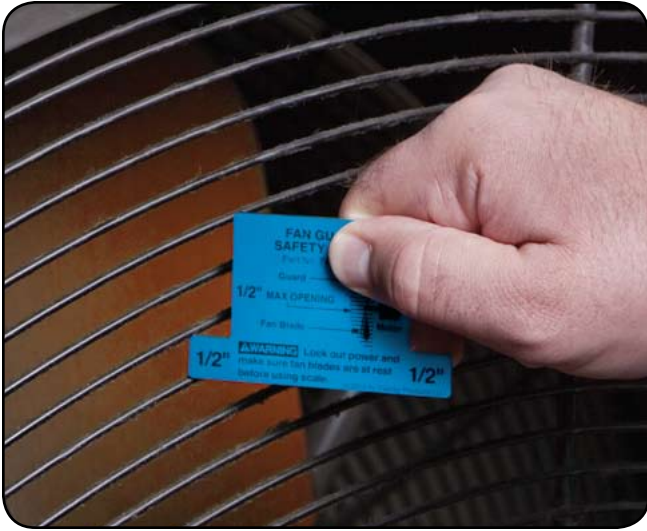
Checking a fan guard that is in compliance.
